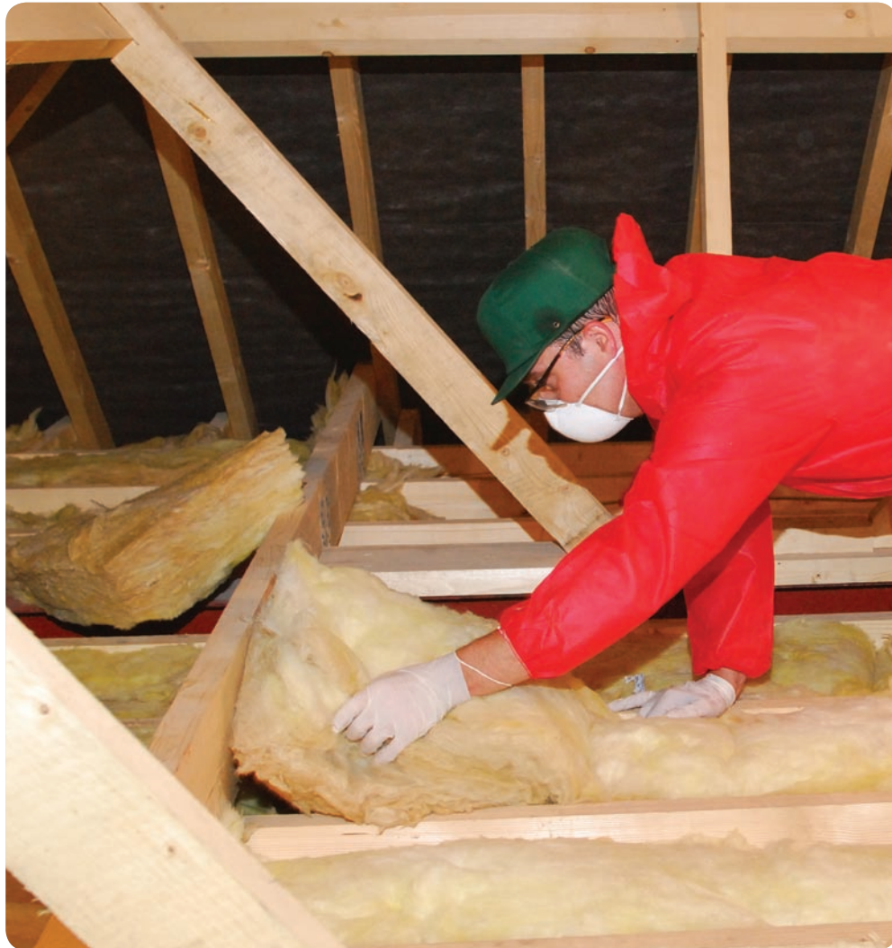
*Image courtesy of National Insulation Association (NIA)
